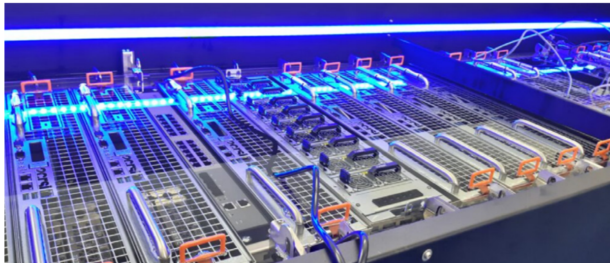
Figure 2. Immersion cooling by Submer
