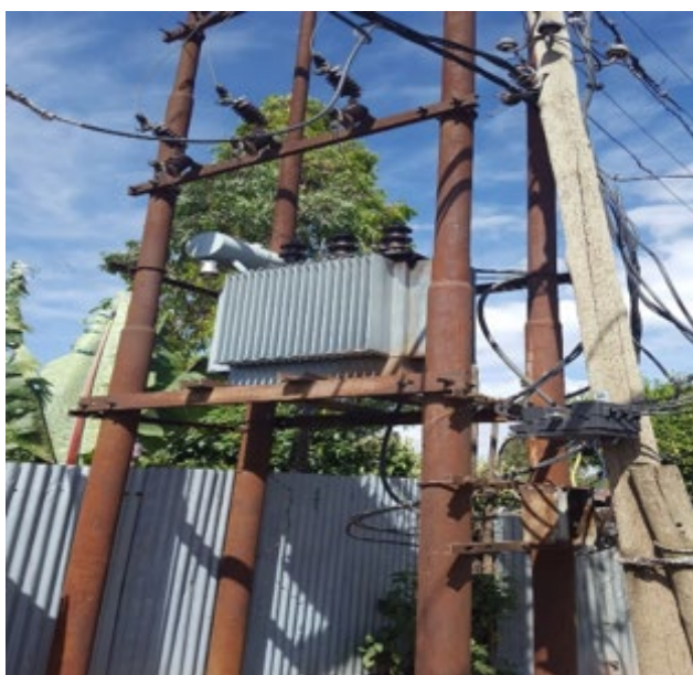
Distribution transformer to be metered for energy balance purposes.
