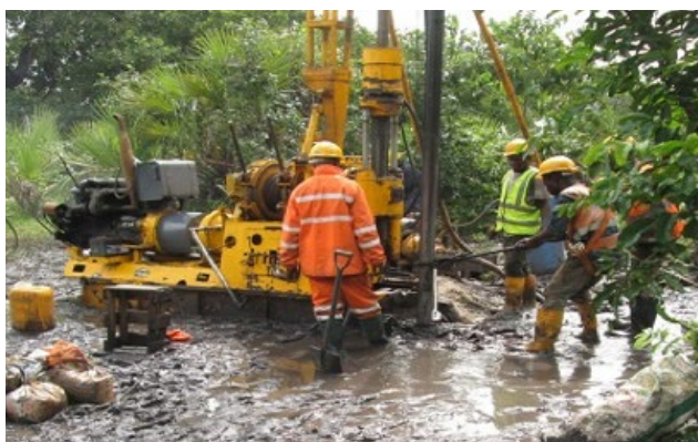
Conducting geotechnical tests at the proposed Somanga site in Tanzania. Photo by PATRP.
