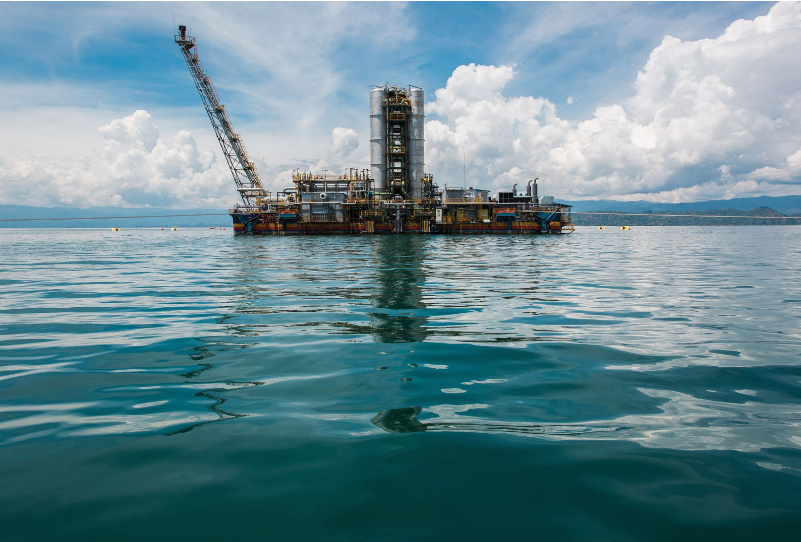
The KivuWatt Power Plant in Rwanda. Lake Kivu is one of Africa's Great Lakes, and straddles the border between Rwanda and the Democratic Republic of Congo. Lake Kivu is a fresh water, volcanic lake, and contains significant amounts of methane gas. Methane can be used as a fuel to generate electricity. Photo by Rachel Couch for Power Africa.
