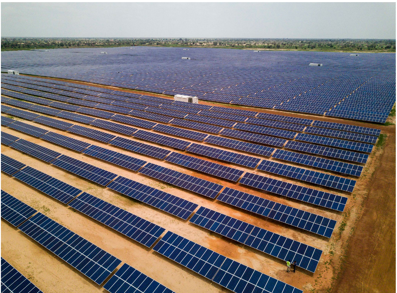
The Senergy I Solar PV plant. Photo by Xaume Olleros for Power Africa.
