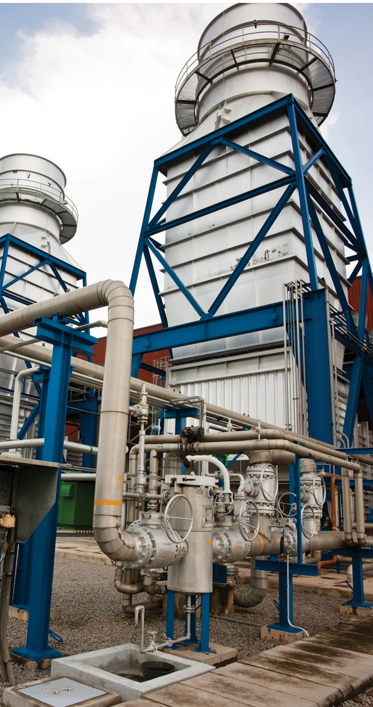
The Azito 288 MW gas-fired generation facility in Côte d'Ivoire uses natural gas supplied from the country's offshore gas fields. Photo by Globeleq.
