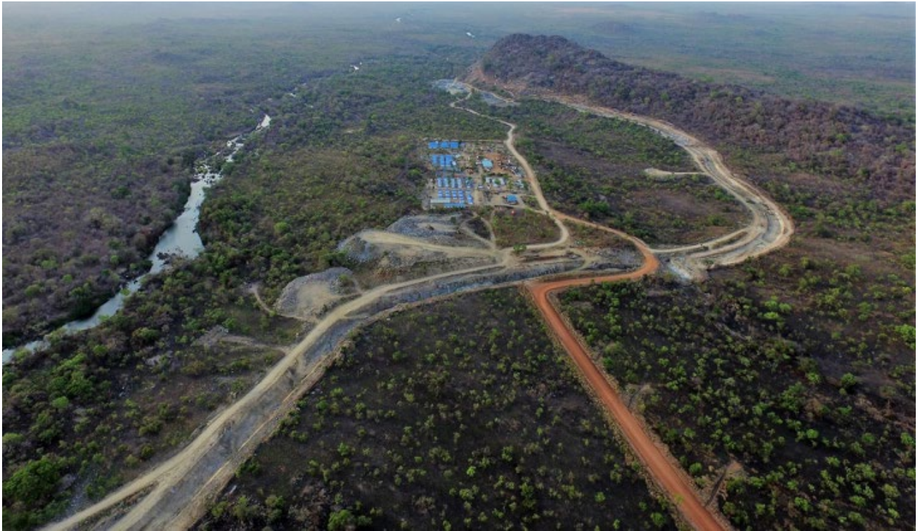
The Achwa 2 Hydropower Project site in Uganda. Photo by ATB Riva Calzoni.
