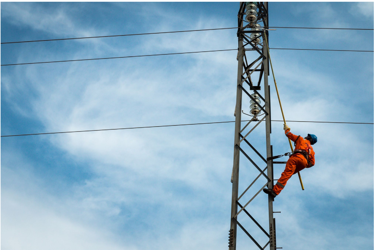
An AEDC linesman climbs an electricity distribution tower to check for faults. Photo by Ryan Kilpatrick for Power Africa.
