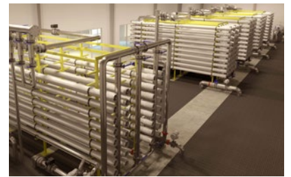
30 MGD Brackish Groundwater Desalination Plant San Antonio Water System, Texas
