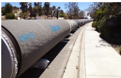
Carlsbad Seawater Desalination Program 54-inch Finished Water Pipeline San Diego County Water Authority, California
