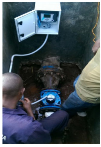
Figure 7: Water Mind Analyzer on DMA bulk meter
