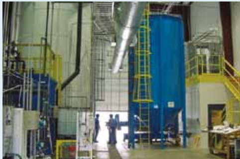
MEMBRANE BIOREACTOR SOLUTION IN CATLETTSBURG, KY
