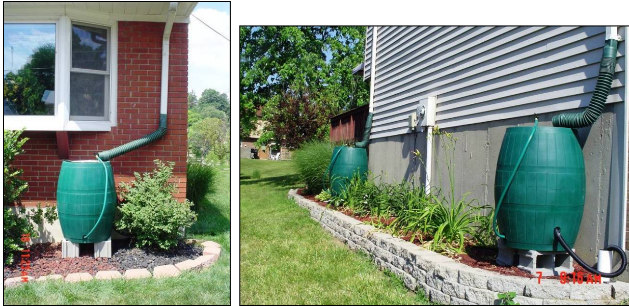
Figure 2 – Photographs of Rain Barrel Installations
