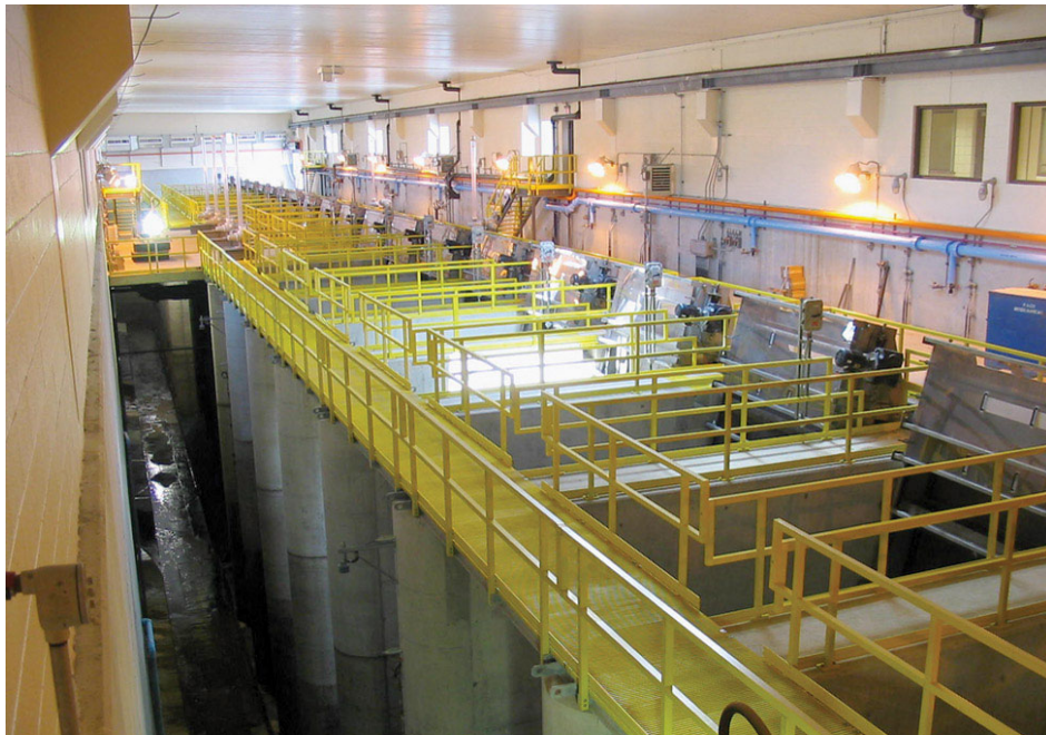
Screening Facilities - George Kuhn Drain CSO Basin Oakland Co. MI, Photo by Tetra Tech
