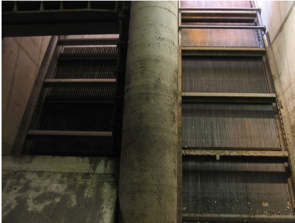
Coarse/Fine Screening - George Kuhn Drain CSO Basin Oakland County, MI, photo by Tetra Tech
