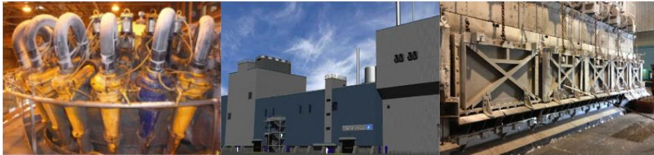
Rio Tinto Alcan, Jonquière Smelter, primary hydrocyclones; Rio Tinto Alcan, Jonquière Smelter, Spent potlining plant EPCM; Rio Tinto Alcan, Kitimat Smelter, furnace repair
