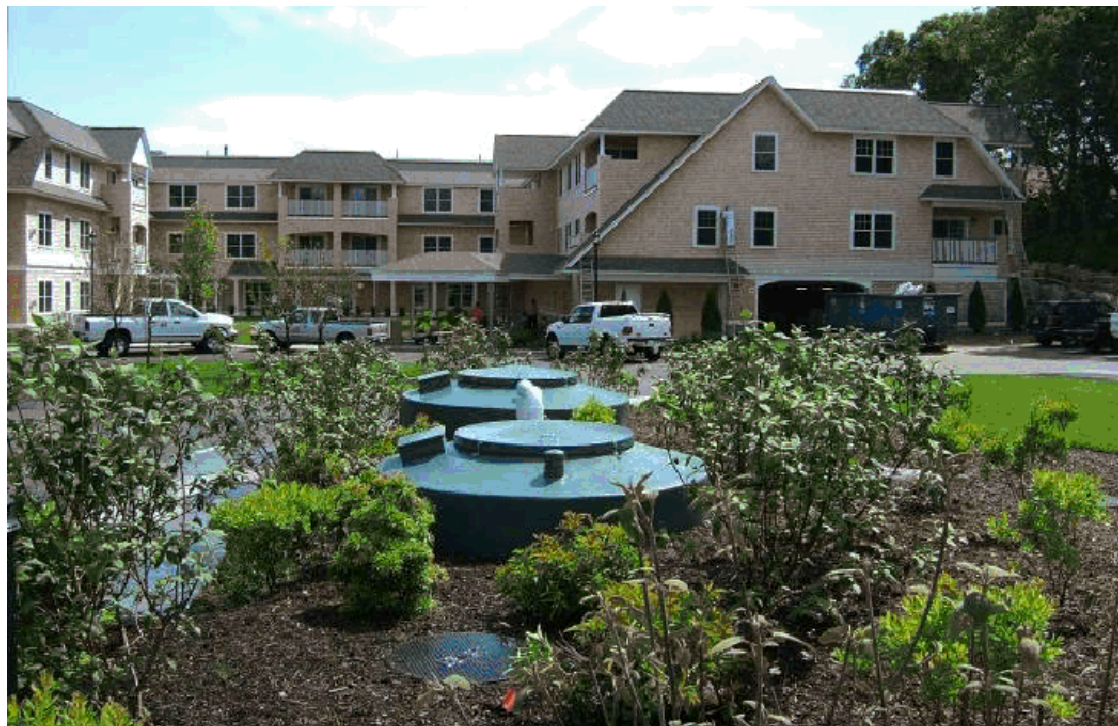
Prepackaged fixed media filtration units such as this one are commonly used to provide affordable and effective treatment in decentralized systems.
