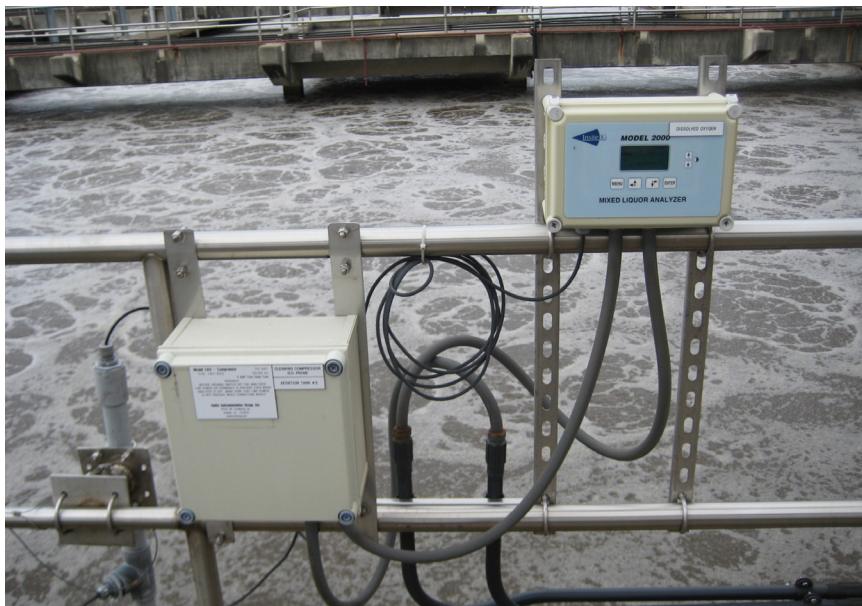
With new controls and sensors, it is possible to hold dissolved oxygen at 1 mg/L, yielding energy savings of 15% to 20%. Tetra Tech
