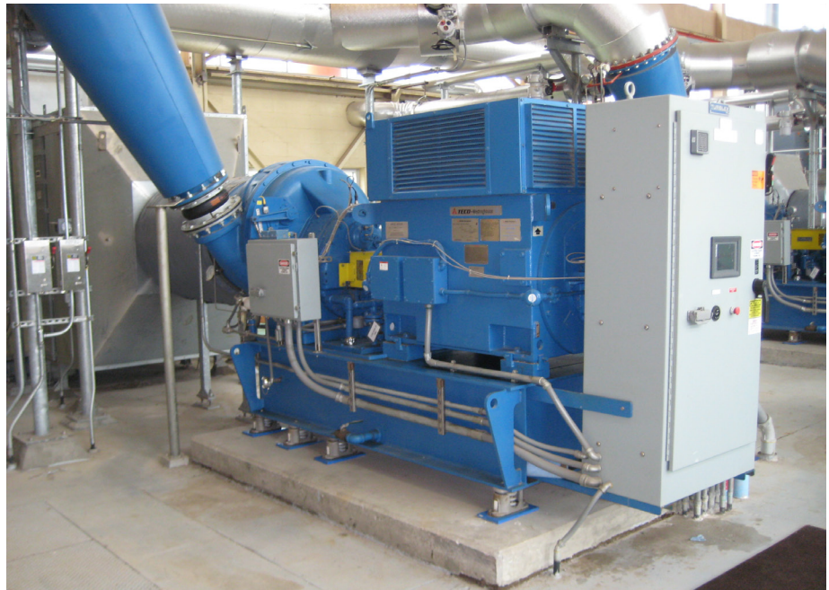
A dual-vane control blower can increase turndown capability. Tetra Tech
